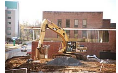
Construction crews work on the parking area outside the future Enrollment Management building at NSU.
